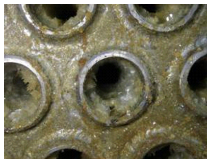
Fig.2 View of pipe blocked by tar
